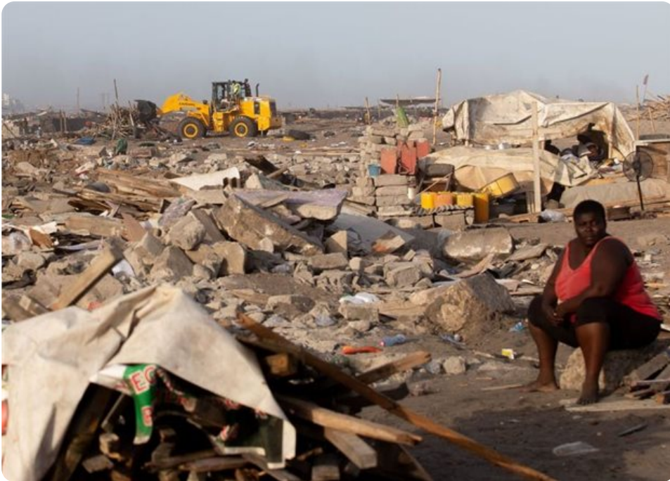
A woman sits at a site in James Town, Accra, demolished in May 2020 to make way for a new fishing port complex. Photo by Nipah Dennis/AFP via Getty Images
